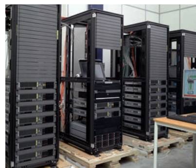
Servers mounted in racks and ready to ship to the site after the emulation sequence
